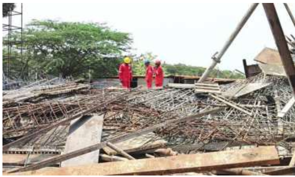
The collapsed portion of an under-construction overbridge at Auto Nagar in Visakhapatnam on Sunday. SPECIAL ARRANGEMENT
